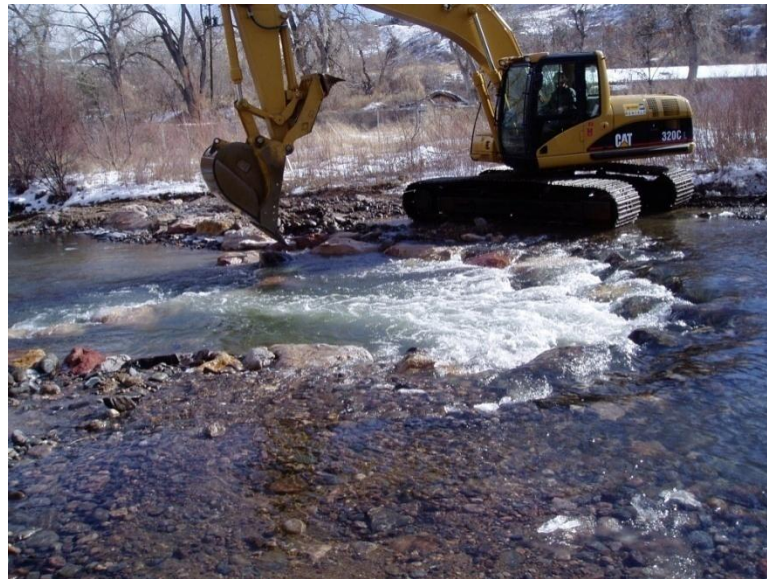
Figure 1. Photograph of a stream restoration project under construction in Clear Creek, Golden, Colorado, showing an excavator placing boulders in a gravel-bed river to control fluid and sediment transport mechanics in order to promote stable fisheries and channel stability
